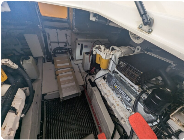
Tiara 4100 Open engine room detail
