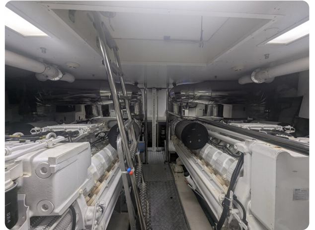
Riva 85 Opera engine room
