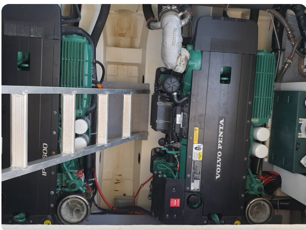
Beneteau MC5 engine room
