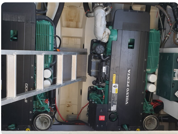
Beneteau MC5 engine room
